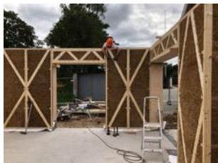
Straw Construction © Henning Larsen Feldballe School is built up of wooden elements of straw that doubles as insulation and structure of the building.
